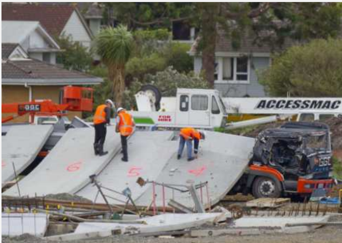
Tornado damage at Hobsonpoint Secondary School Construction site
